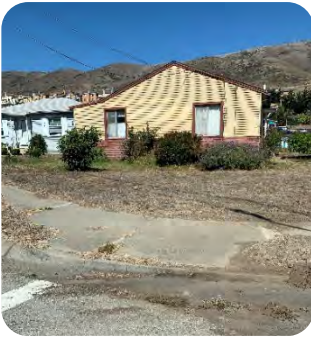
Figure 19 – Non-compliant Curb Ramps in South San Francisco
