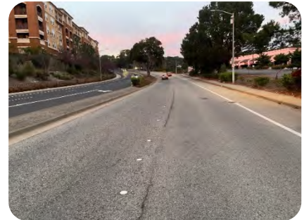
Figure 16 – Gellert Blvd Surface Seal Candidate
