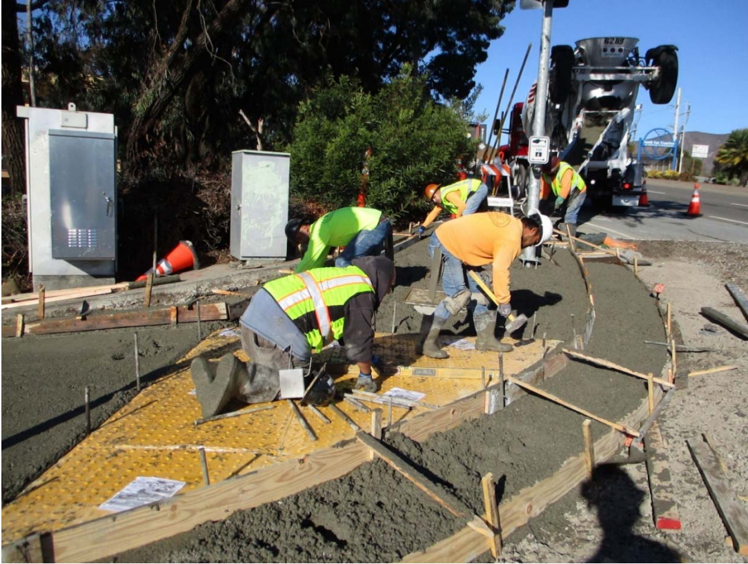
Photo 9: Construction of concrete sidewalk and curb ramp at the southwest corner of E Grand/Grand Ave
