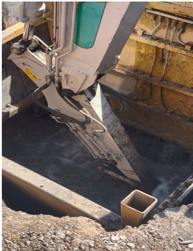
Photo 6: Encountering large amount of water intrusion during the traffic signal foundation installation
