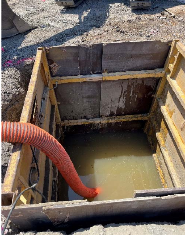
Photo 5: Encountering large amount of water intrusion during the traffic signal foundation installation
