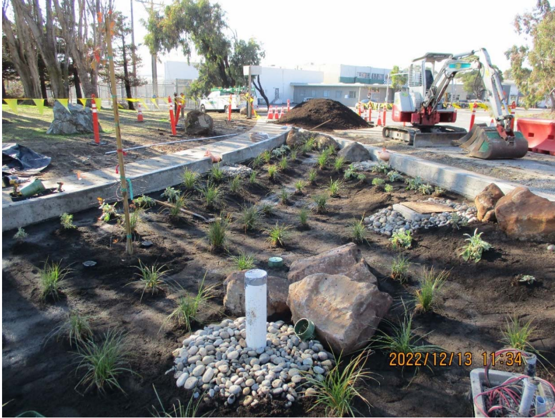
Photo 3: Construction of the new biofiltration area at the southeast corner of E Grand/Grand Ave
