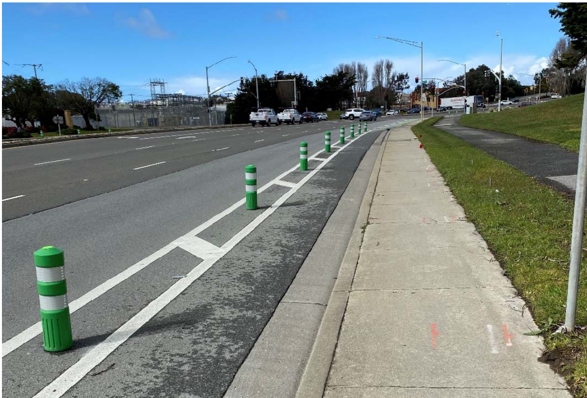
Photo 12: Installation of new protected bicycle lane with delineators along E Grand Ave
