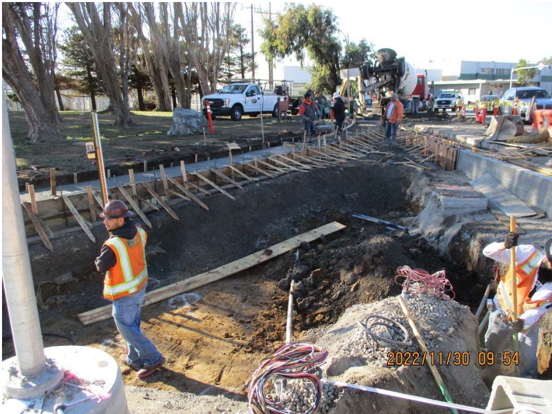
Photo 2: Construction of the new biofiltration area, sidewalk, and curb/gutter at the southeast corner of E Grand/Grand Ave
