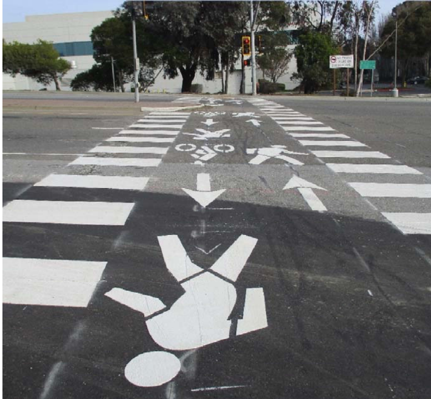
Photo 13: Installation of new enhanced pedestrian and bicyclist crossing at the west leg of the E Grand/Grand Ave intersection
