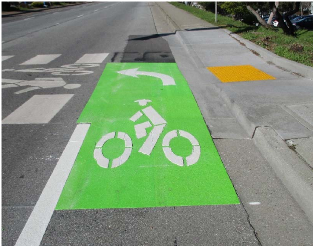
Photo 14: Installation of new green bicyclist box at northwest corner of E Grand/Grand Ave
