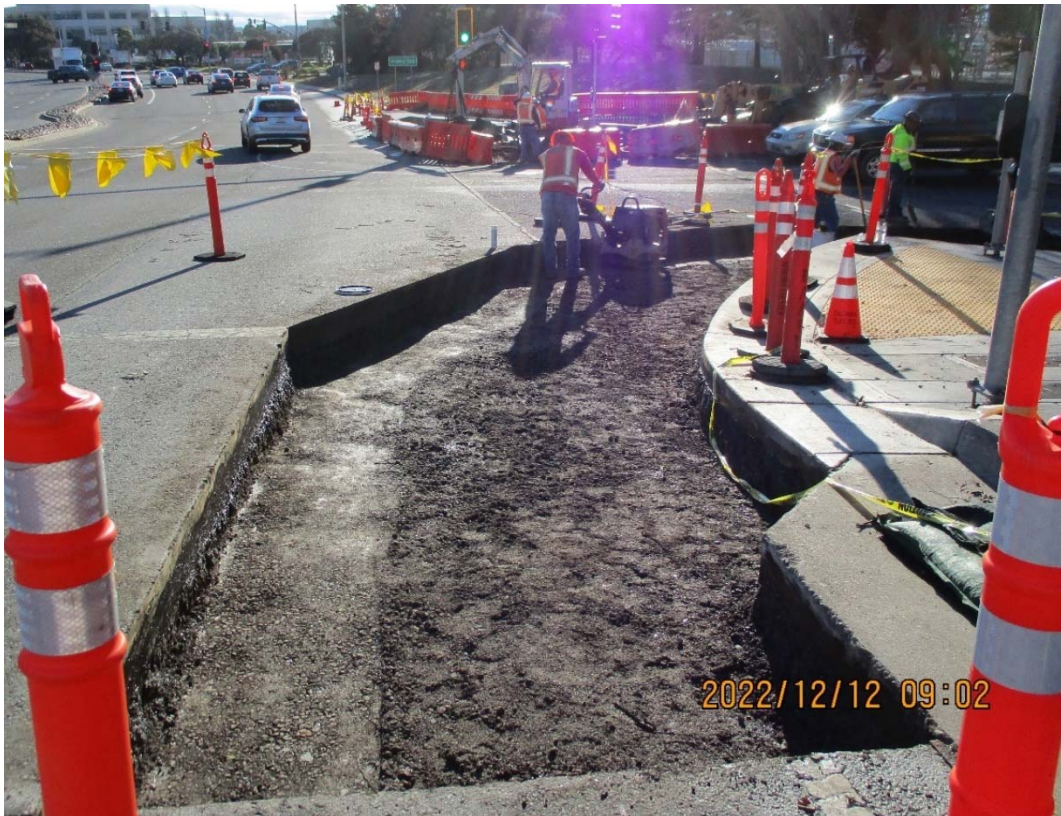
Photo 10: Construction of street paving to conform with new curb ramp and sidewalk at the southwest corner of E Grand/Grand Ave
