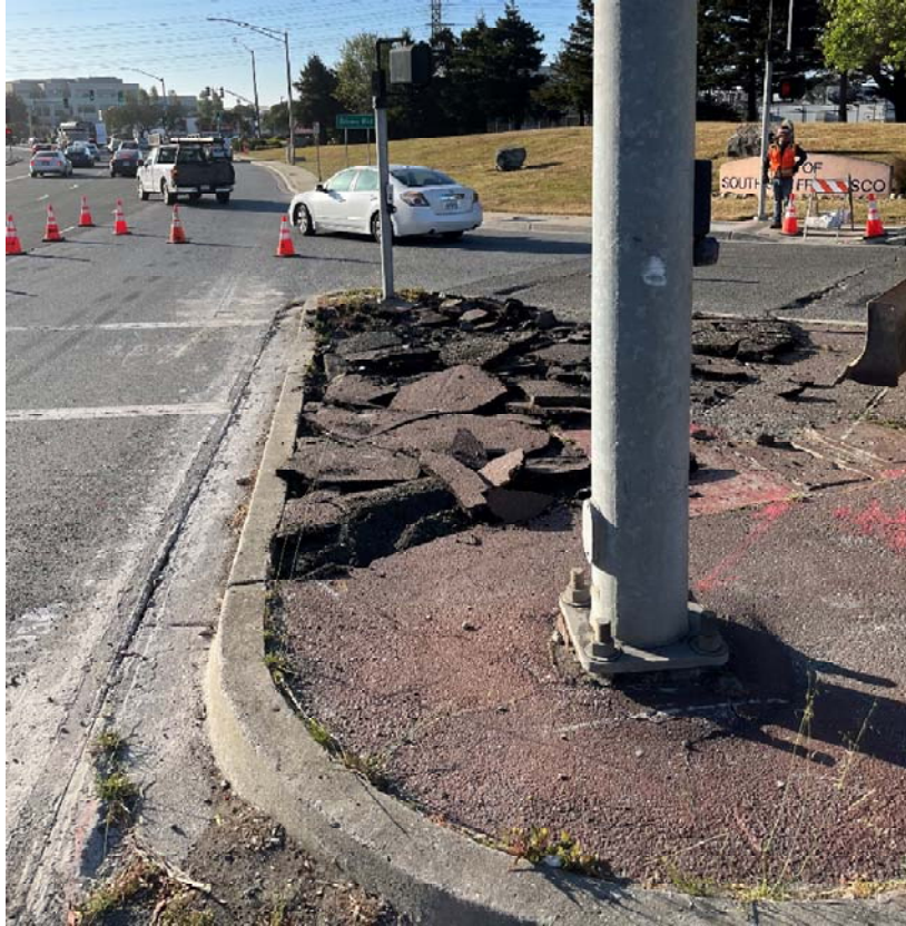
Photo 1: Demolition of the island at the southeast corner of E Grand/Grand Ave
