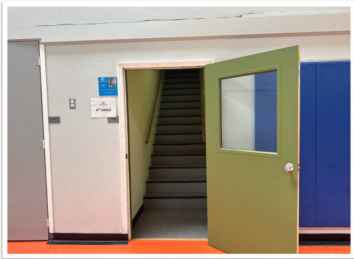
8th grade classroom not ADA compliant/wheelchair accessible
