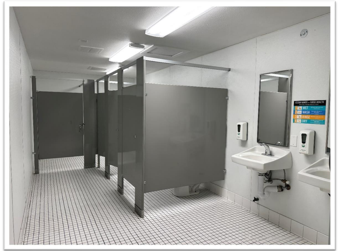
Student bathrooms - constant plumbing issues No easily accessible staff bathroom
