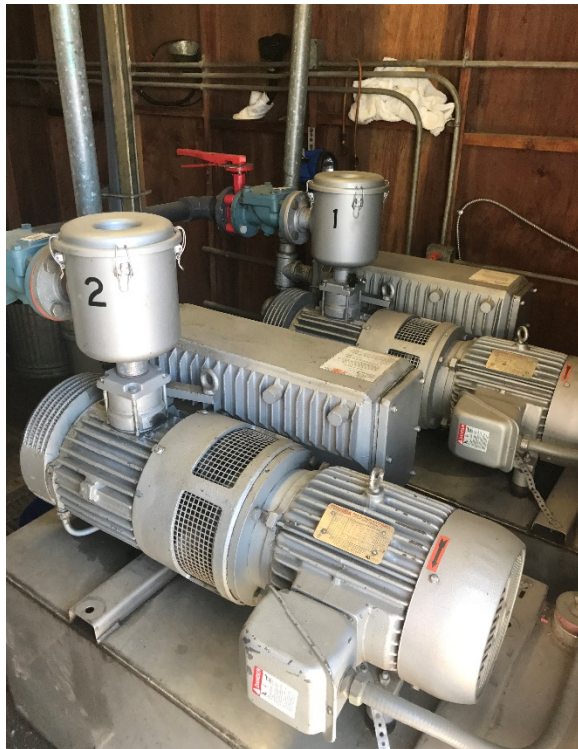
Figure 1 Existing vacuum pumps located within the pump house.
