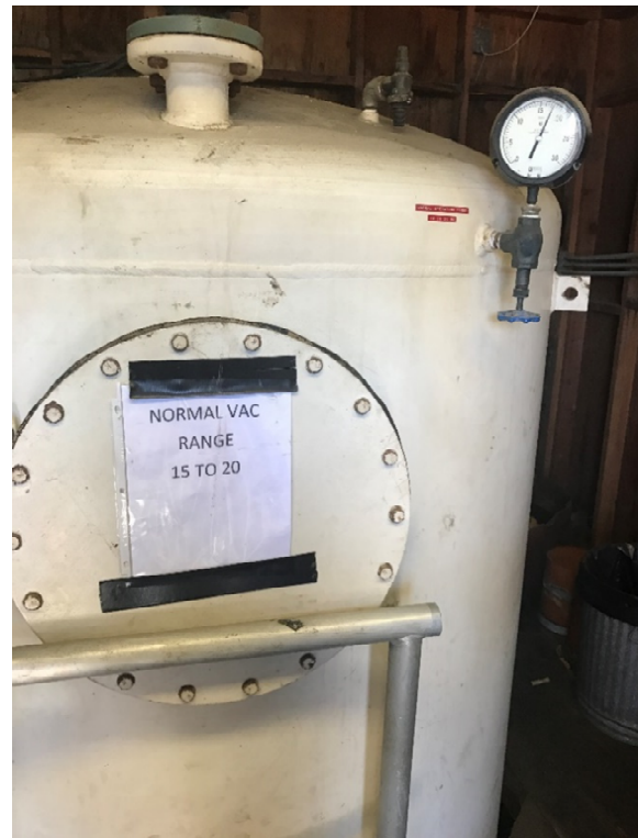
Figure 2 Vacuum tank located within the existing pump house.
