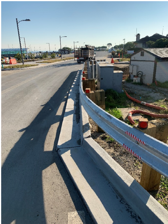
Figure 3 Existing switchgear in the center with the vacuum/ejector pump station on the right. The realigned Marina Blvd. is to the left, roughly 4 to 5-feet higher in elevation.
