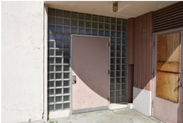
Figure 13. Flush wood door surrounded by prismatic glass block, at east elevation. Partially boarded-over flush wood door at south elevation pictured at right, looking northwest.
