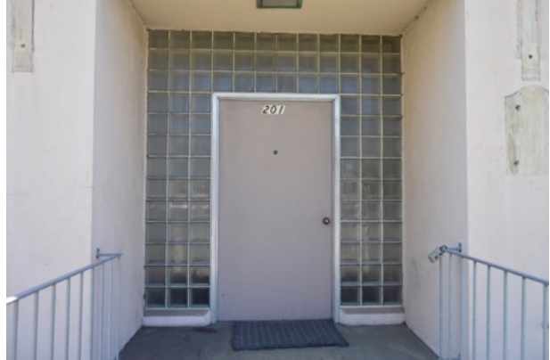
Figure 6. Recessed entrance with flush-wood door and glass block surround at facade, looking south.
