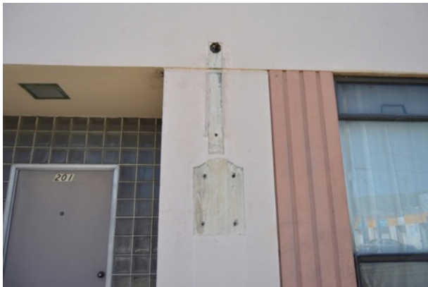
Figure 7. Missing exterior feature to immediate west of entrance, looking south.
