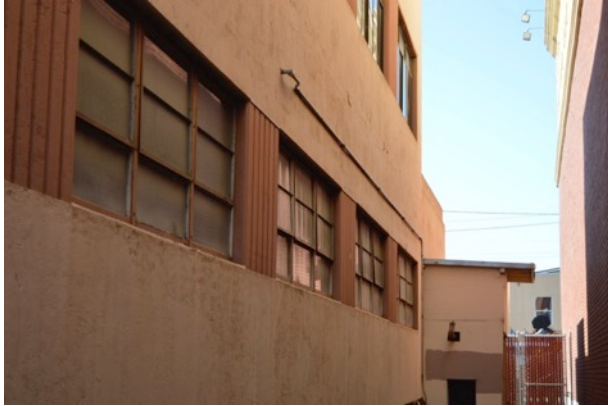
Figure 18. Steel windows located along first story of the west elevation. Shed roofed addition pictured in background, looking south.
