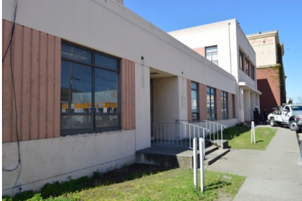
Figure 5. Windows, fluted concrete details, and entrance at east end of facade, looking west.
