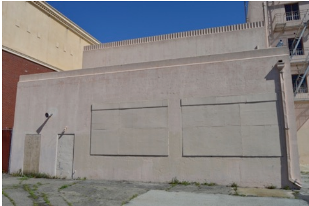
Figure 15. Infilled and boarded-over door and window openings at west end of south elevation, first story. Standard replacement windows at second story.
