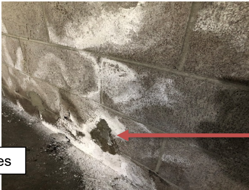
Fig 15 – Retaining Wall Efflorescence
