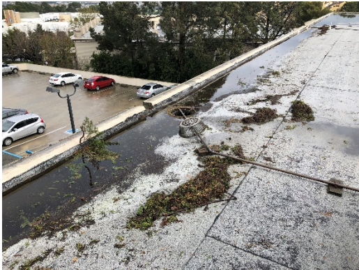
Fig 17 – Debris and Ponding on Roof
