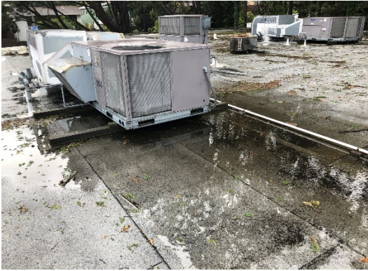
Fig 18 – Sleepers Across Roof Drainage
