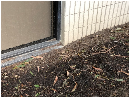
Fig 25 – Dirt at Foundation Window
