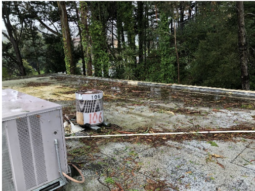
Fig 16 – Debris and Ponding on Roof
