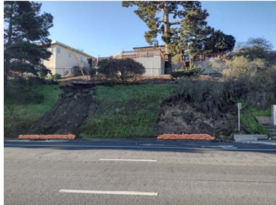
Photo 10. El Camino Real embankment failure
