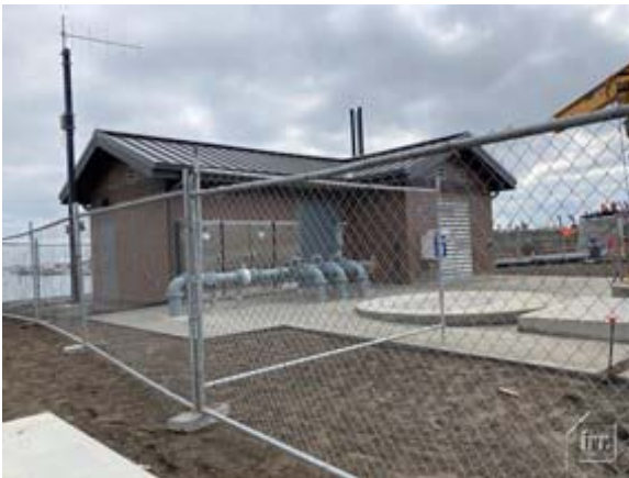
Sewer Pump Station
