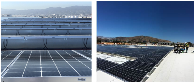
Solar Panel Distribution Main Campus; Panels on PS2 and T5
