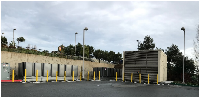
New Nitrogen tank for the South Campus next to B42
