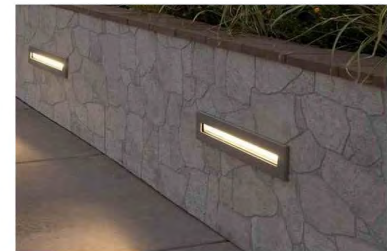
Courtyard and Rooftop: Recessed Wall Light by BEGA Lighting
