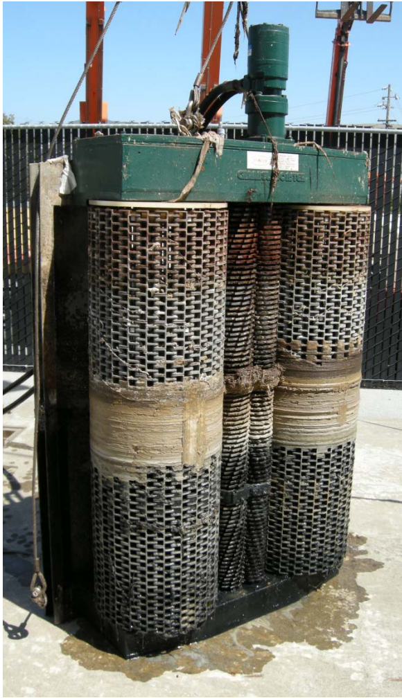
Sewage Grinder Before Refurbishment
